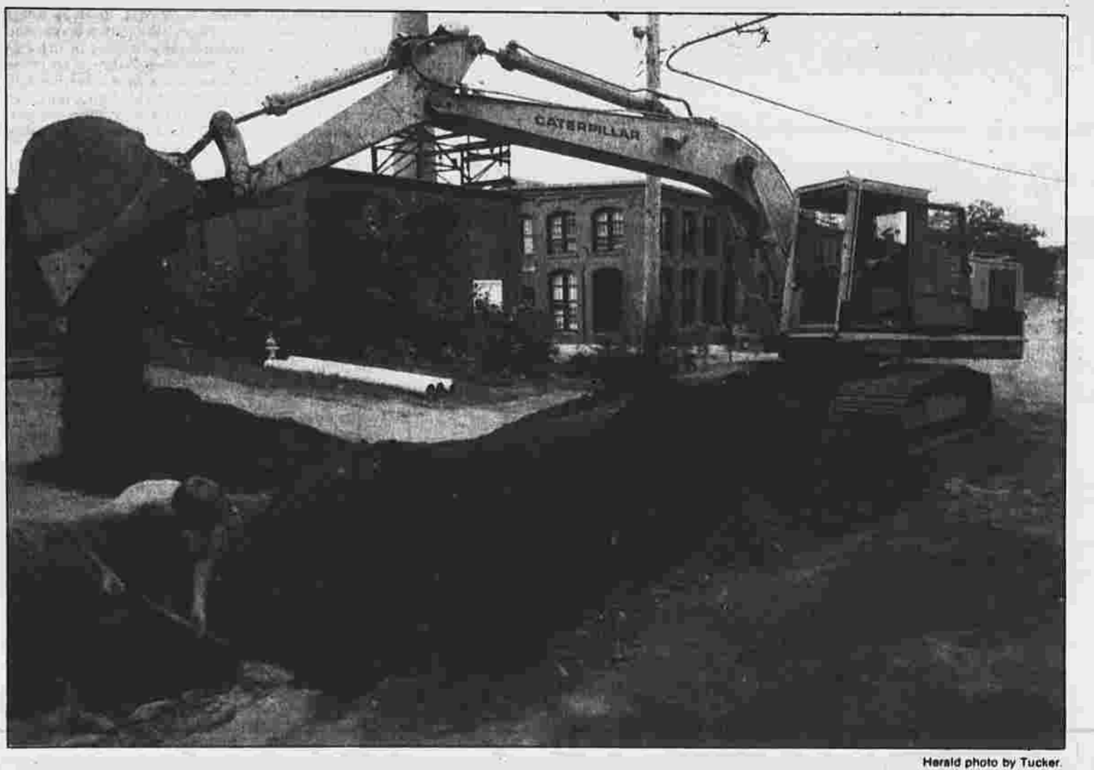
The Milton C. Beebe Co. of Storrs is currently completing utility work - the first step in improvements being made in Manchester's Cheney Historic District. This excavation is on Forest Street, with the Clocktower Mill - one of four being converted to apartments - in the background. The Beebe workers are Glen Burnham of Storrs at left and James Forand of Mansfield, operating the backhoe.
